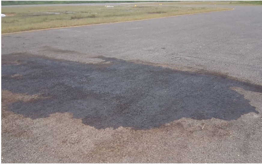
Figure 4: Fuel spill on the aerodrome apron
