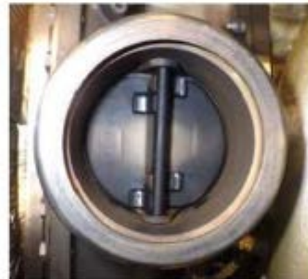
Photo No. 9 P2.7/P3 Check valve
