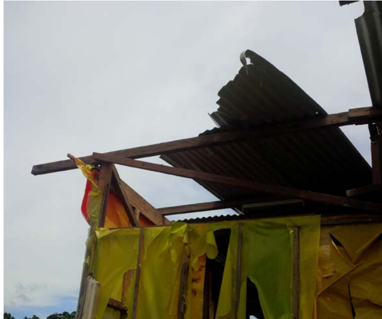
Figure 3: Damage to generator shed roof
