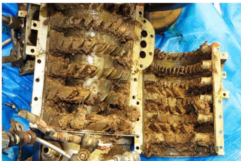
Figure 30: Split-line bolts removed, exposing mud and grass
